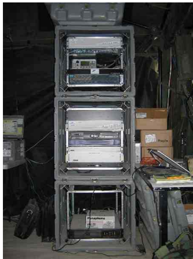
Master Reference Terminal Electronics
