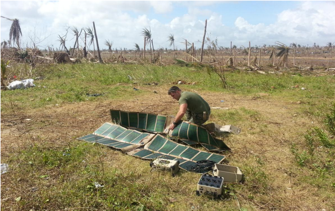
Fig 3 – Bren-Tronics Solar Power System in Guiuan, Philippines
